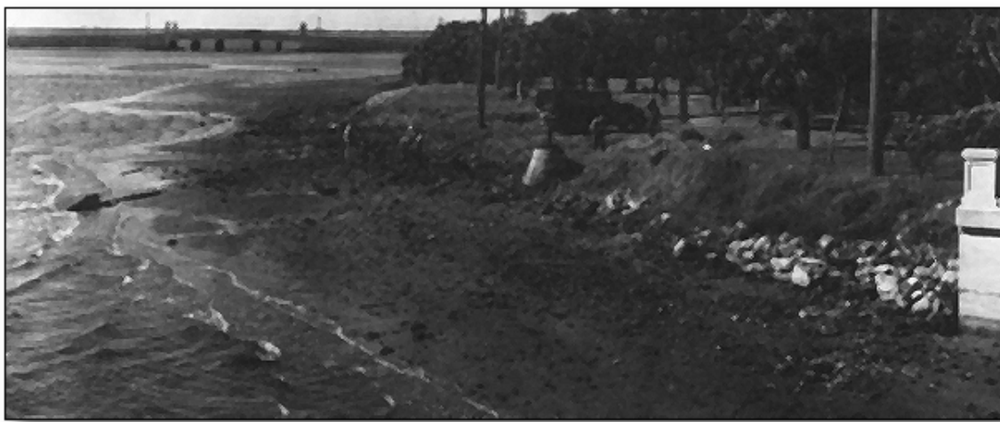
Before assistance came from Washington under the New Deal, the city of Tampa provided public service jobs. These workers employed by the Tampa Cooperative Council on October 24, 1932 were building a retaining wall along Bayshore Boulevard in Tampa. Later, the WPA completed the project.
